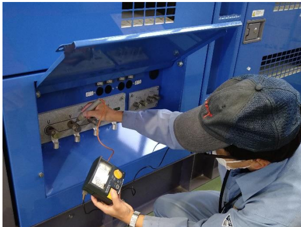
Measuring insulation of generator
