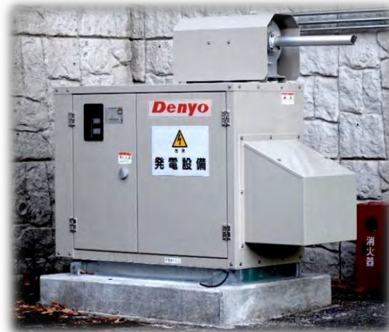
In-house generators installed in hotels for use in the event of disaster
