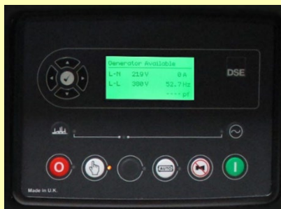
MANUAL & AUTO - START GENERATOR CONTROLLER (DSE7310MK II)
